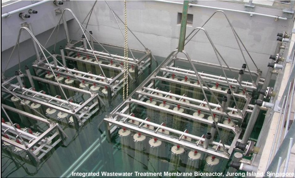
Integrated Wastewater Treatment Membrane Bioreactor, Jurong Island, Singapore
