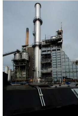
Sembcorp Biomass Power Station, UK
