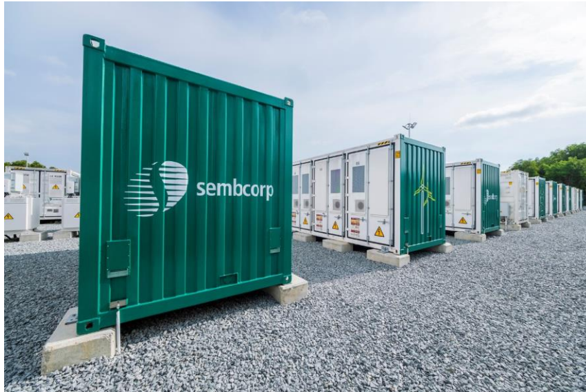
Sembcorp Industries successfully commissioned Southeast Asia's largest Energy Storage System of 285MWh on Jurong Island within six months.
