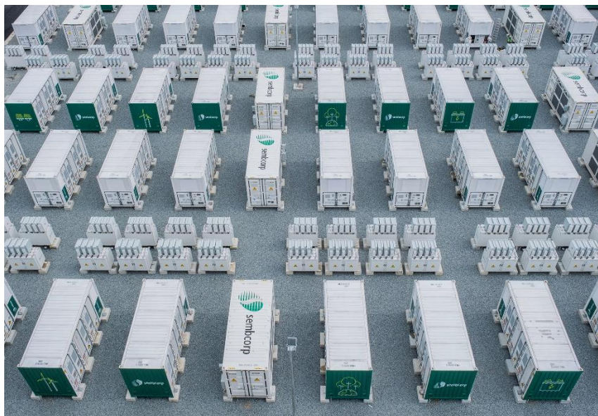
With the contracted capacity to store and deliver 200MW of power for one hour, the ESS will be able to meet the daily electricity needs of nearly 17,000 four-room Housing & Development Board public housing flats in a single discharge.
